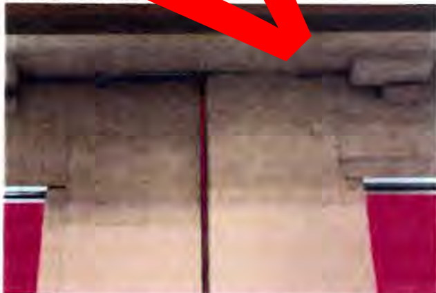
Image showing gap where double doors meet at top
