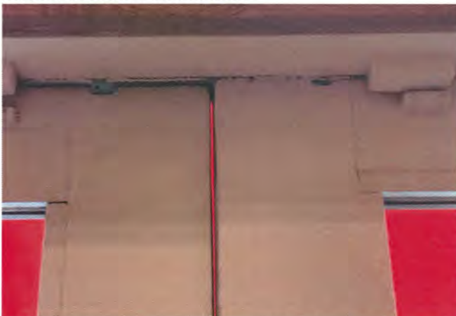
Image showing gap where double doors meet at top
