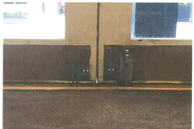
Image showing gap where double doors meet at bottom
